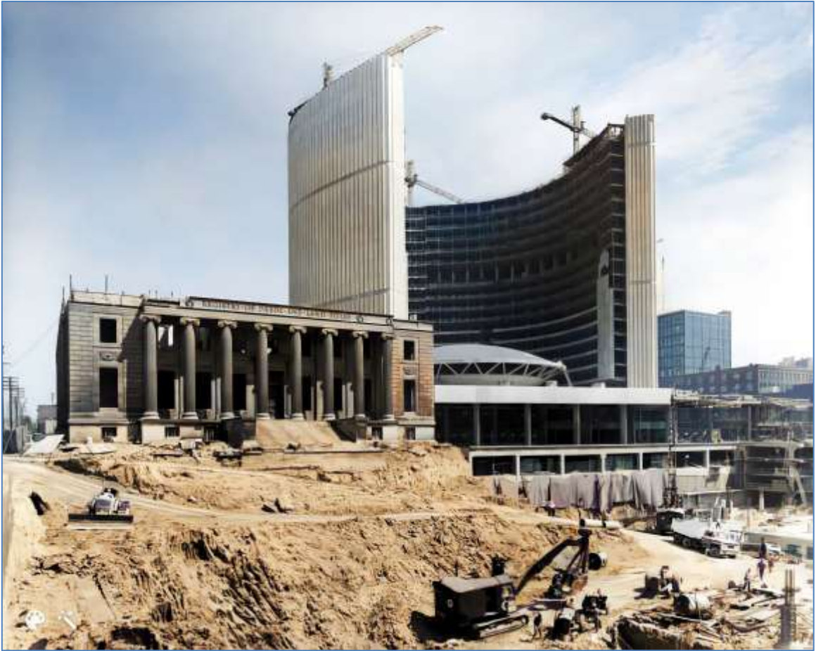
“New” City Hall was under construction in 1964, with the Registry of Deeds and Land Titles building still on the left. City of Toronto Archives
